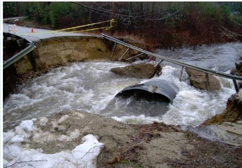
Culvert failure on Blake Brook in Epsom
