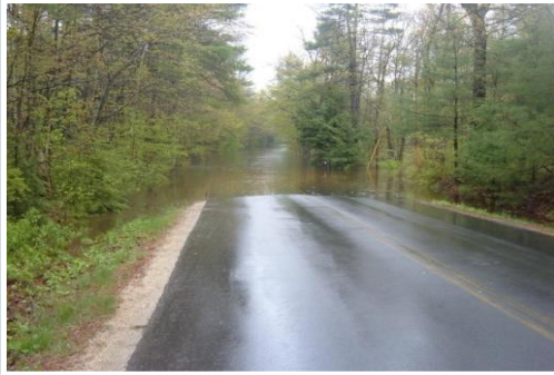
Water overtops a culvert in Lee and the river crosses the road
