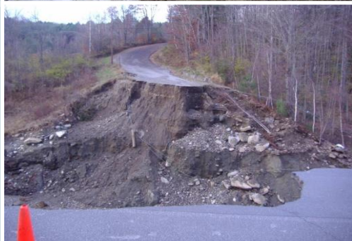
Catastrophic culvert failure in Alstead lead to loss of life
